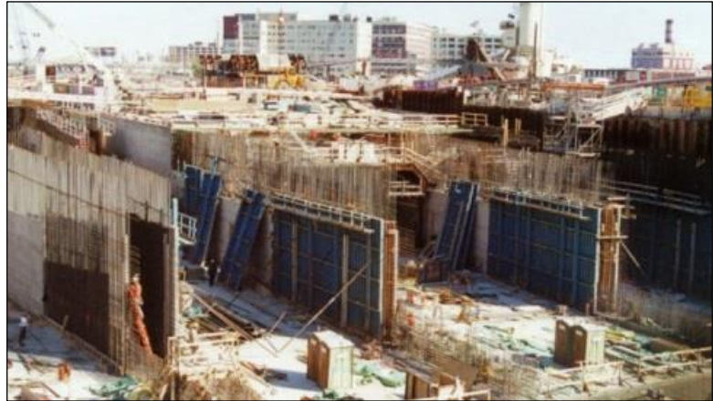
The construction of O’Neill Underground Tunnel. Tons of dirt were excavated, the tunnel was constructed of concrete, and then overlaid with elements of the Rose Kennedy Greenway.
